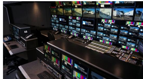
36HDX Production – Kayenne Switcher
